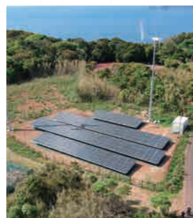
Takushima Energy Farm
